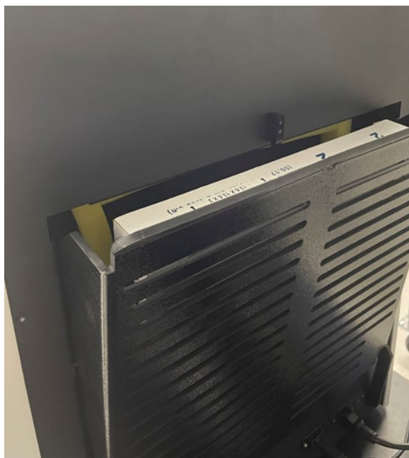
Figure 19. Air filter cover opened with air filter exposed.
